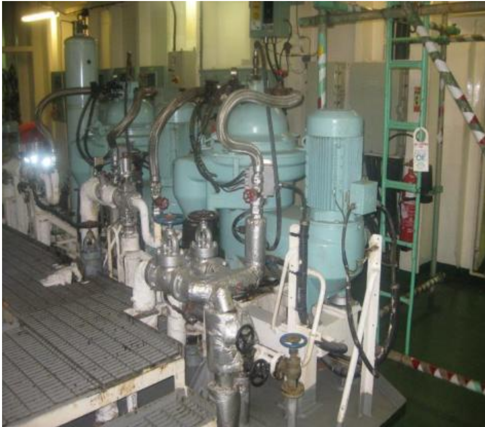
Figure 6.3: Typical purifier systems on-board
